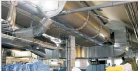
In the first expansion stage, the ceiling mounted exhaust air heat exchanger has already saved about EUR 8,000 per year.
